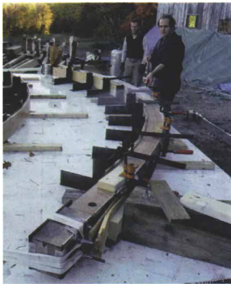
After the steamed timber was clamped into place on the bending table, Levin hosed it down to keep it from checking.
